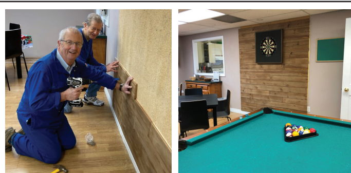
Norman Picton and Howard Gray continue renos on our Mission. Seen here refurbishing the dart board wall. No labour costs and supplies purchased inexpensively. Great job – well done! Thank YOU.
